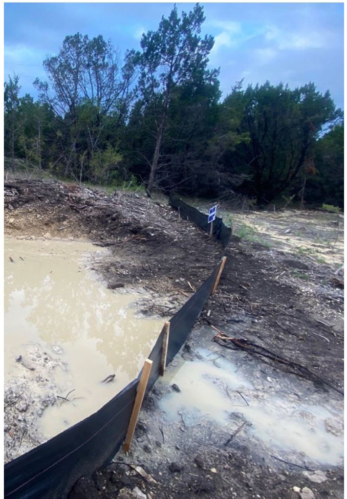
Construction of a pipeline in Central Texas' Hill Country created erosion and runoff in May 2020.
